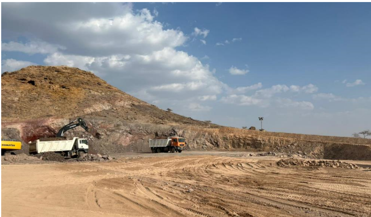
Image 2: First cut mining activities and overburden and limited oxide copper ore removal
