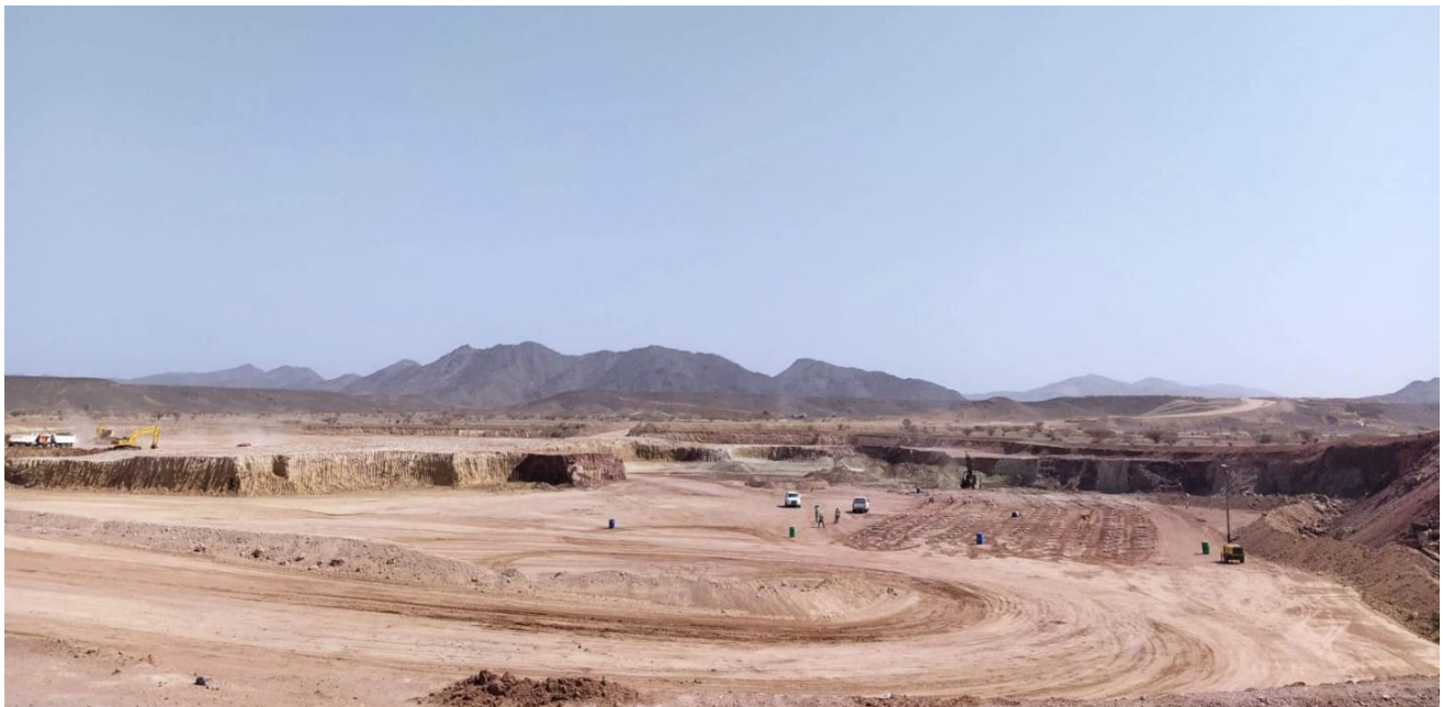
Looking north - picture showing 0-year pit area; top layer removal in progress
