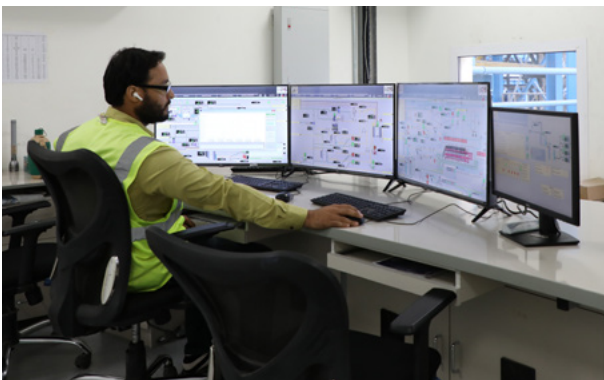
Plant control room
